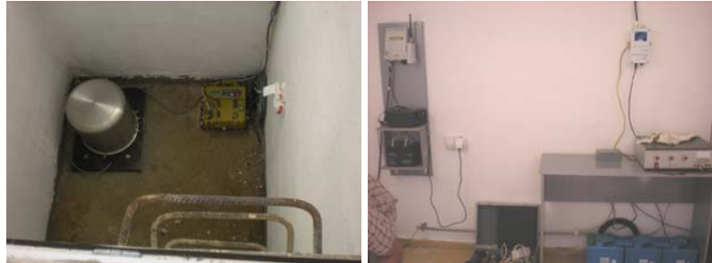
Dracevica seismic and geodynamic station: fully equipped weak, strong motion and geodynamical station with professional microwave wireless link
